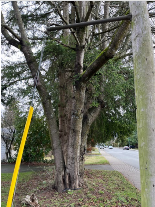
Photo 7. View east of City Cherry 7642/523 shared with property owner. It has 3 included stems from base. The northern stem (523) is leaning to the site.
