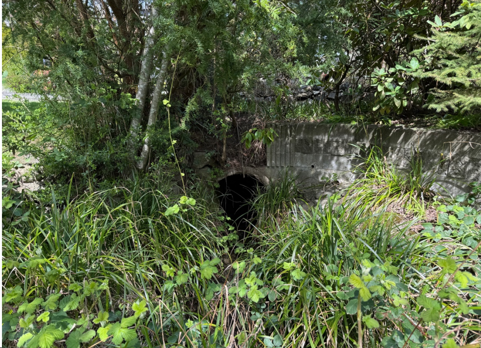
Photo 1: Upper extent of the stream looking north at the storm sewer outfall on the south side of Malabar Ave.
