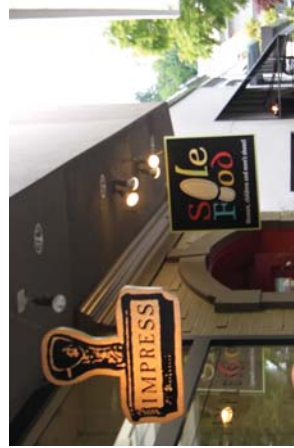
Unacceptable: externally illuminated sign face. Exposed suspension wire/ cables from canopy and poor example of exposed lighting soffit fixture.
