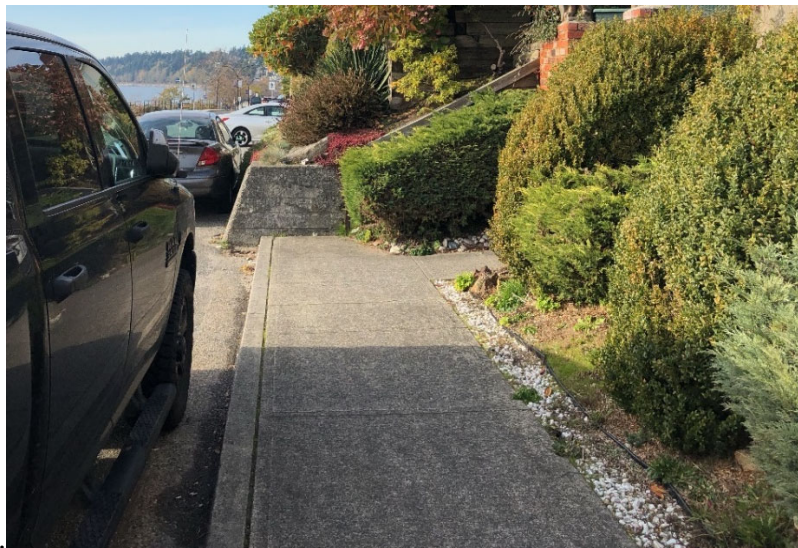
Example of a sidewalk in White Rock that ends at an encroachment.
