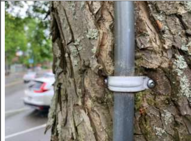
Photo 9. View of Honey Locust #34 tag 3103 with electrical conduit being encompassed by tree trunk. Majority of lights within crown require removal prior to pruning.
