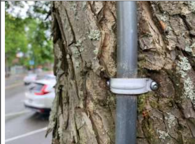
Photo 9. View of Honey Locust #34 tag 3103 with electrical conduit being encompassed by tree trunk. Majority of lights within crown require removal prior to pruning.
