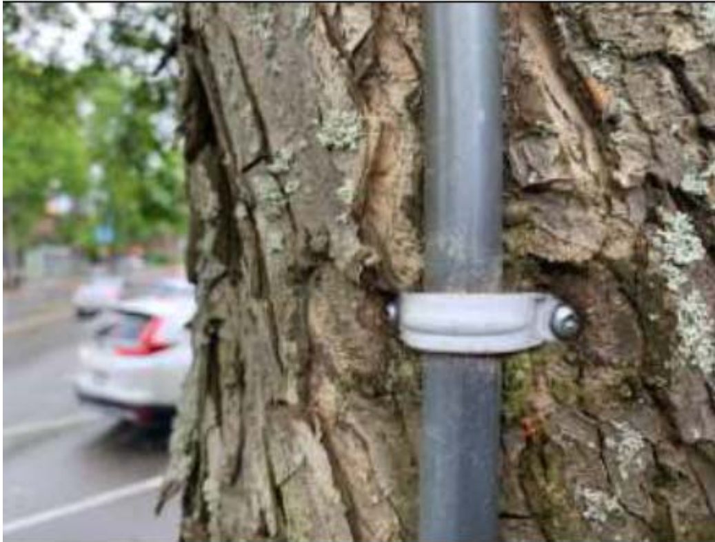
Figure 4: Electrical Conduit in Tree Trunk – Johnston Road south of Prospect Avenue.
