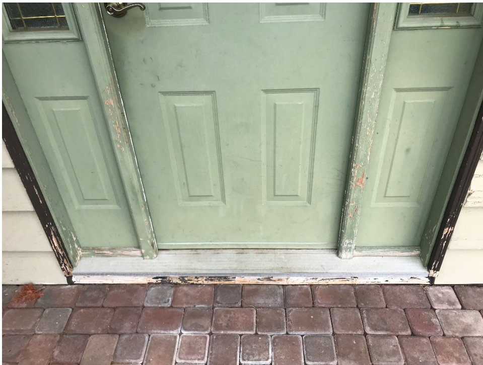
Exterior Paint Defects
